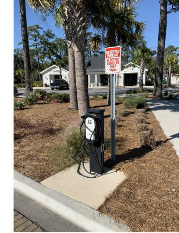
EV CHARGING STATION
