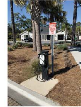
EV CHARGING STATION
