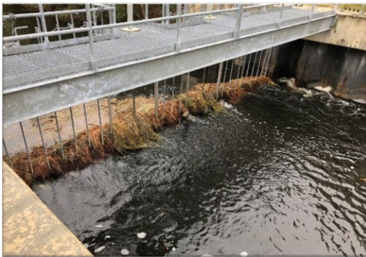
Hurricane Irma Vegetation Blocking Intake Chamber
