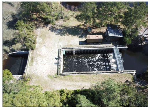
Wexford Pump Station
