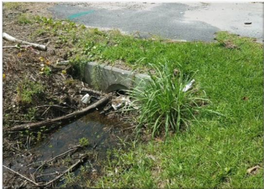
Drainage Issue on Katie Miller Rd
