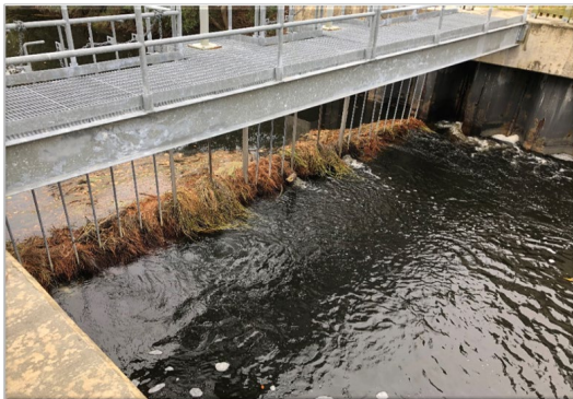
Hurricane Irma Vegetation Blocking Intake Chamber
