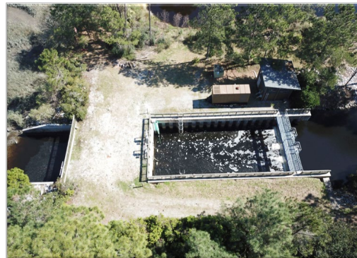
Wexford Pump Station
