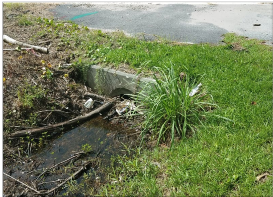
Drainage Issue on Katie Miller Rd.
