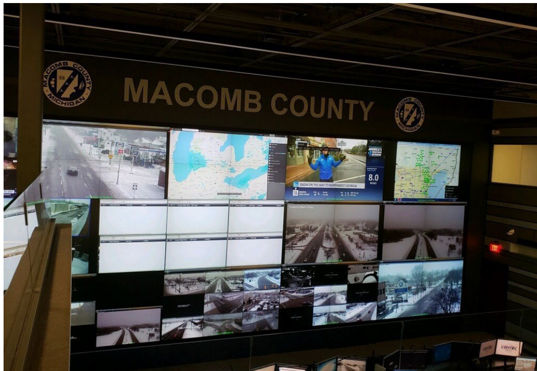
Traffic Signal Monitoring
