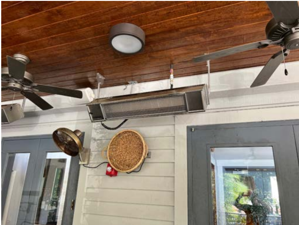
Image 6: Existing exterior heater
