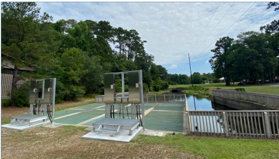
The Jarvis Creek Pump Station at full capacity can pump 44,000 gallons of water per minute.
